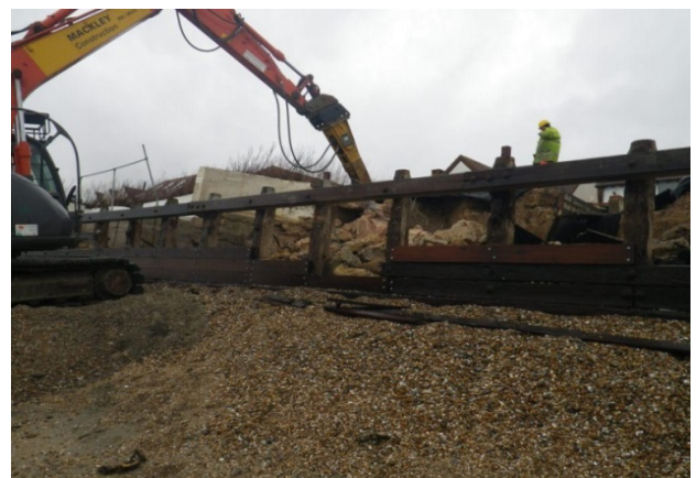
4. Breastwork failure at East Wittering as a result of undermining due to low beach levels 6 th January 2014
